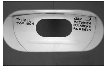
This is what the deck-to-bulkhead joint looks like before the hull is trimmed. The deck is unsupported and will not have a good bond with the bulkhead.
